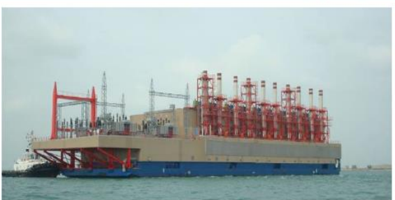
Power Barge Conversion for KPS Alican Bey
